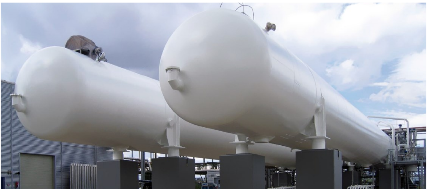
Figure 5.6: Cylindrical LH 2 tanks at the hydrogen liquefier in Leuna, Germany. Source: Linde
