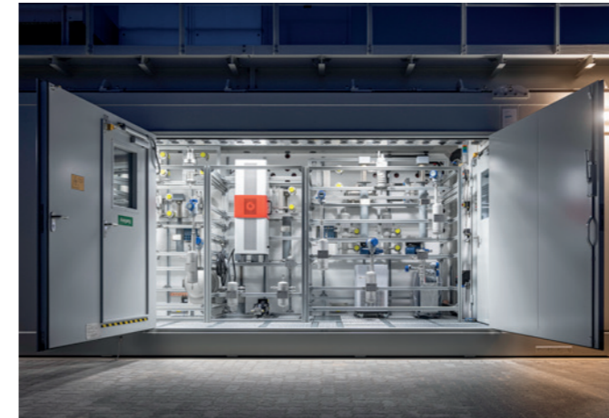
Electrolyzer container from the KIT – Karlsruhe Institute of Technology
