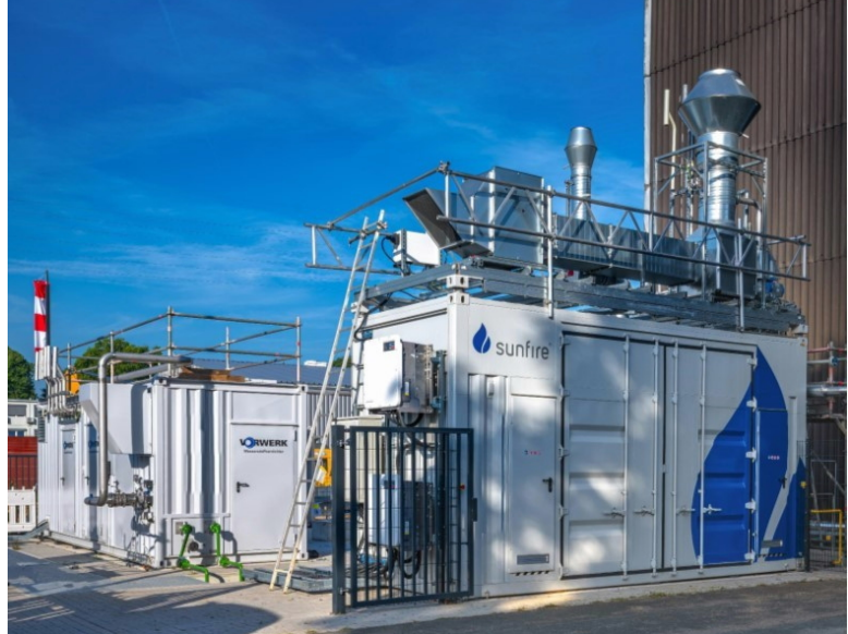
Operating 250 kW high-temperature electrolyser. Source: RWE Generation SE
